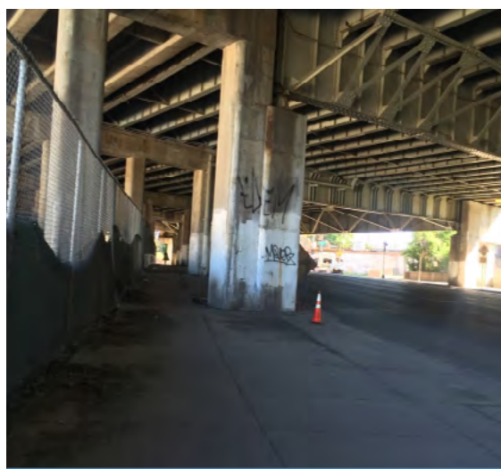
Existing sidewalk along Ashland Avenue (looking north) from the 606 trailhead, connecting to the Clybourn Metra. | See Page 79 for ideas on potential improvements.
